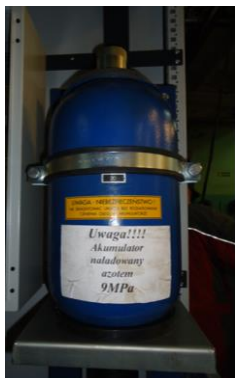
→ Hydraulic Accumulator for Emergency Fast Operations
